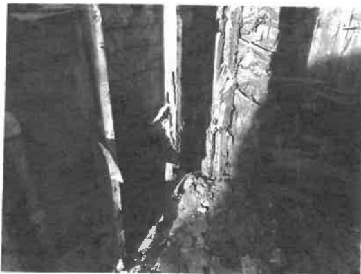
ROTTEN STUDS AND SHEATHING
